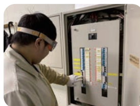
Emergency power shutdown
