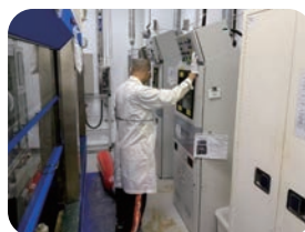
EMO activation for gas cylinder cabinet
